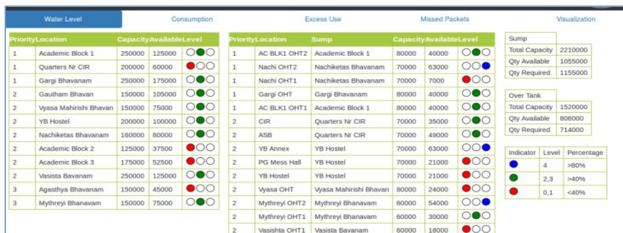
Fig.3 Screenshot of Web Interface for Smart monitoring system
