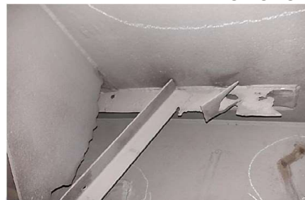
Figure 14 Degradation by corrosion of the brackets of tubes of gauging
