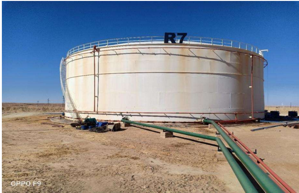
Figure 05 Crude storage bin
