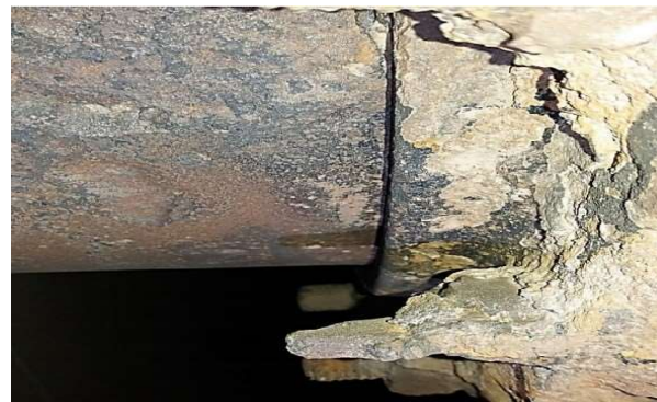
Figure 13 Degradation by corrosion of the flange of their line shipping side back
