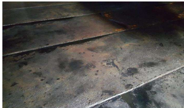
Figure 19 the sheet metal of bottom R8 Before there repair
